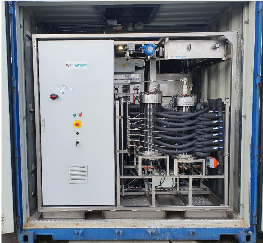
Figure 4. Final EHP sub-system integrated into the container of HyGrid system at HyGear.
