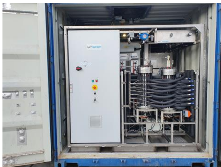
Figure 4. EHP sub-system skid installed in the HyGrid system at HyGear
